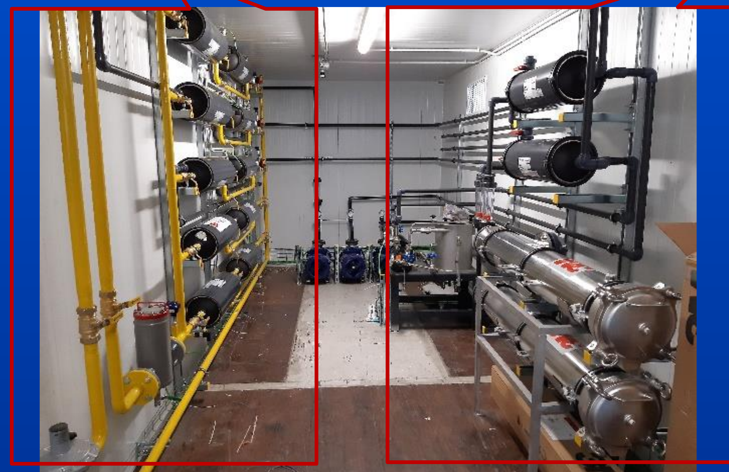
Figure 4: Biogas upgrading and CO 2 recovery parts
