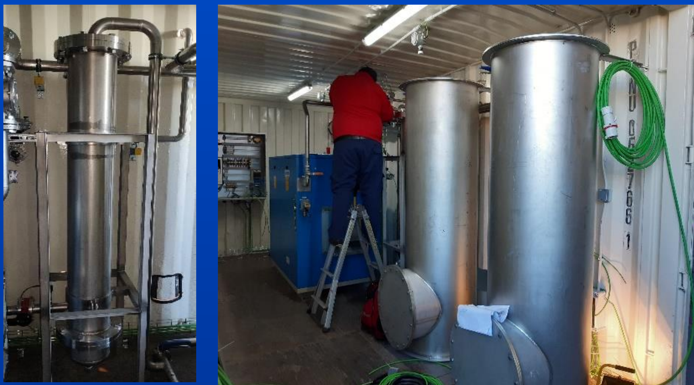
Figure 3: Condenser and activated carbon tanks
