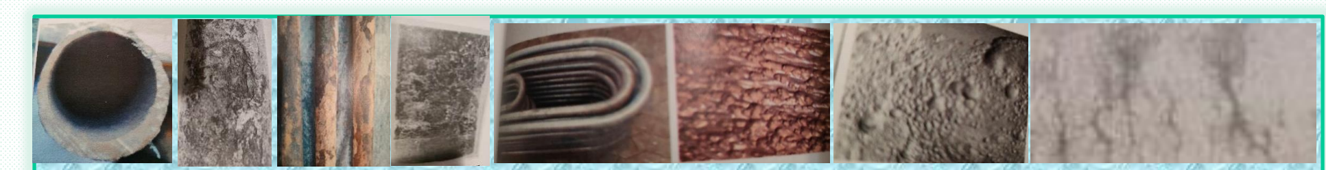
Figure 3 Root causes of boiler tubes failures including scale inside the heat exchanger and deposits formation around the heat exchanger tube (at the top). Effects on Boiler tubes thinning, scabbing, pitting, Flow Accelerated Corrosion and cracking (at the bottom)
